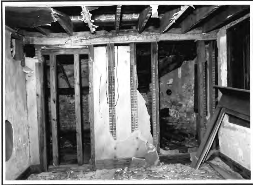
Figure 18. Matthew Jones House, original rear plate of house, now supported by modern framing and carrying 1893 joists.
