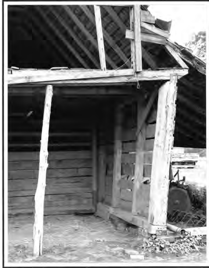
Figure 25. Gray Farm Barn (recently disassembled), detail of rear wall. These large oak posts were originally hole set. The bottoms of the posts were cut off and a sill installed in 1922. (Photo credit: Willie Graham, Colonial Williamsburg Foundation.)
