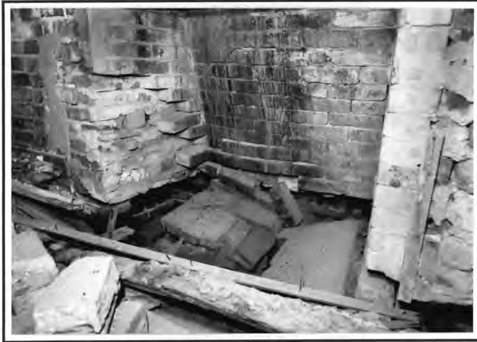
Figure 47. Matthew Jones House, detail showing deterioration in west fireplace.
