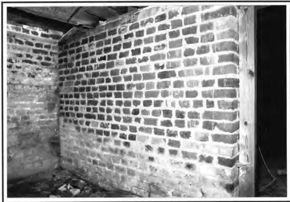
Figure 44. Matthew Jones House, foundation wall built under wall between the shed and main block of the house. This feature was added in 1893, likely when the floor joists were cut and new ones installed in the main block.
