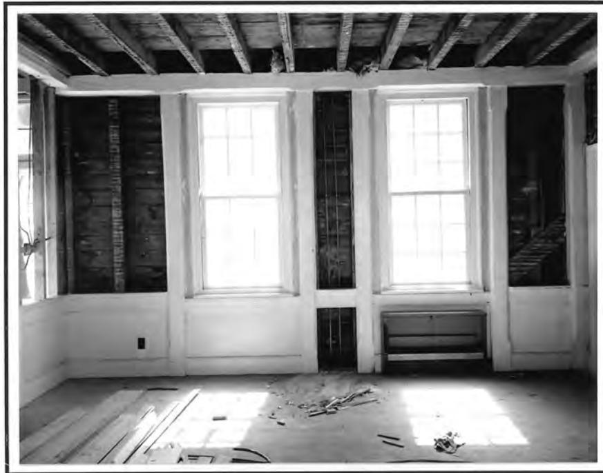
Figure 21. Belle Air, interior wall elevation. As at the Matthew Jones House, the partition to left does not intersect the longitudinal wall at a major post. (Photo credit: Mark R. Wenger, Colonial Williamsburg Foundation.)
