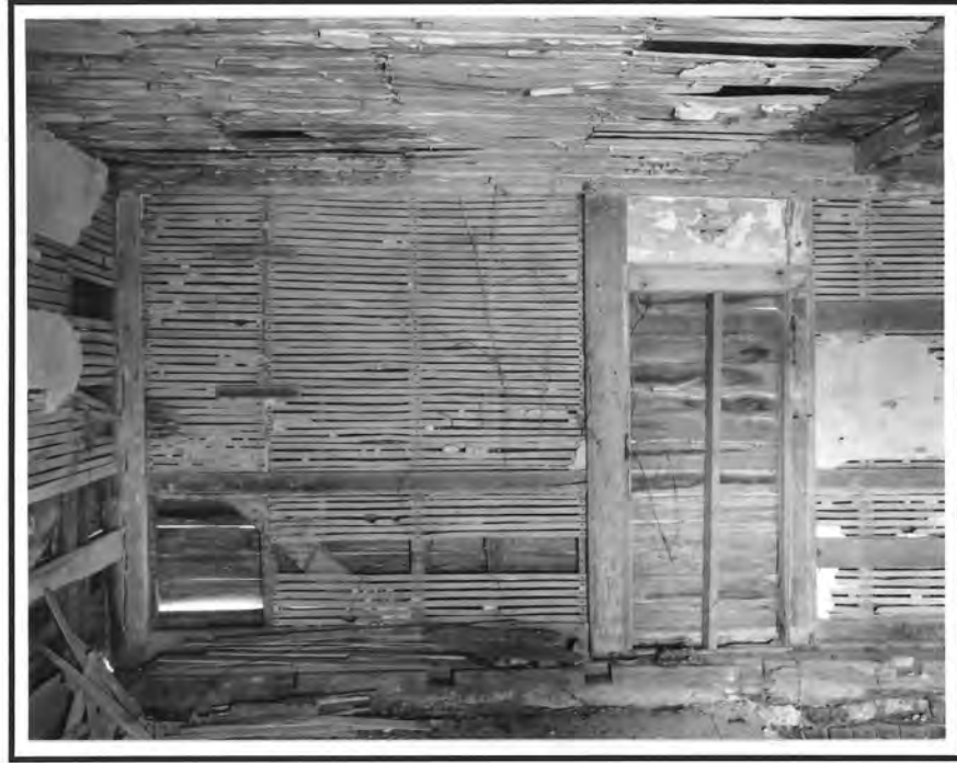
Figure 20. Pear Valley, original front wall. Note the exposed plate, corner, and door posts. The ceiling was originally exposed as well, and later was plastered. (Photo credit: Willie Graham, Colonial Williamsburg Foundation.)
