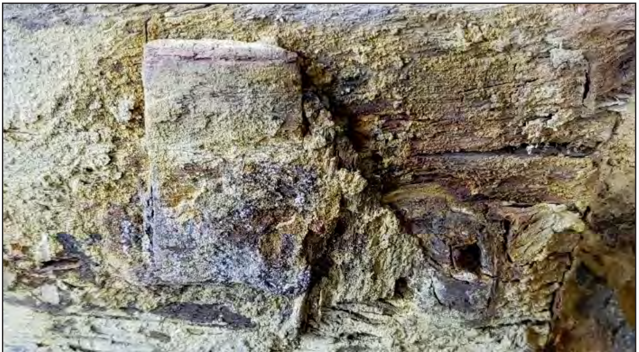
Figure 6.87. Block in the bottom of floor timber FL-12 and plank spike hole.
