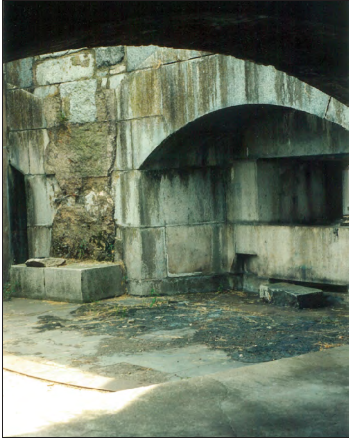
Figure 3.19. Interior of a casemate at Fort Wool, 1990 (photograph by J. Charles, courtesy of Michael Cobb).
