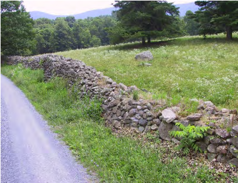
Figure 18. Road frontage walls at western edge of Perna property. Apart from the section in the foreground much of the wall is in good condition.
