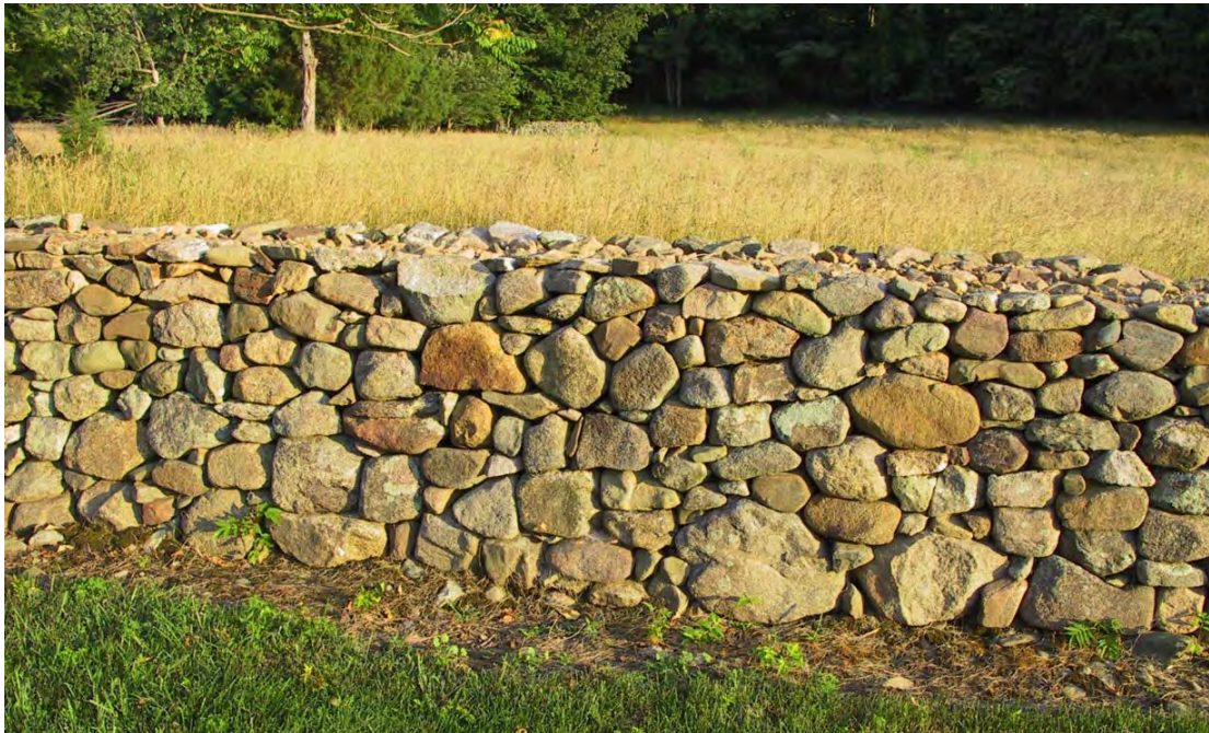
Figure 72. Face of wall rebuilt by Clem brothers showing tightly fitting face stones.
