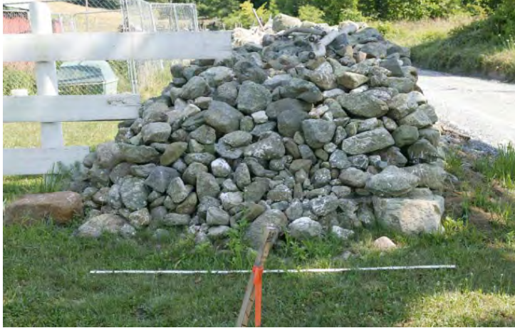
Figure 50. Collapsed northern end of roadfront wall on south side of driveway, looking south.
